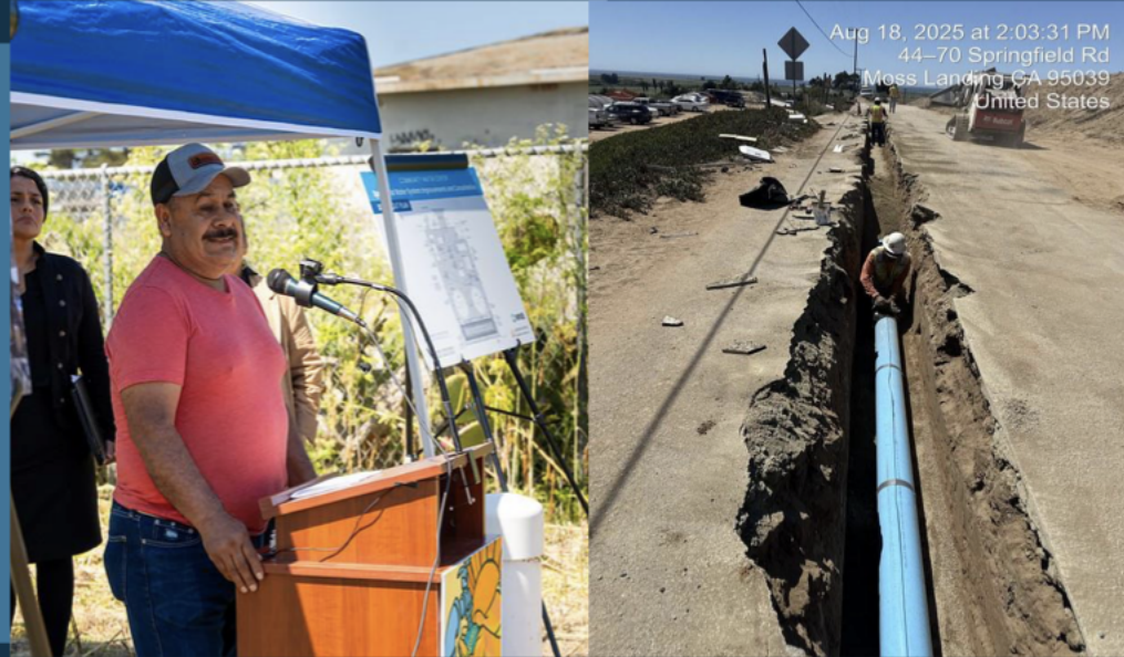
Community Leader speaking at the project groundbreaking in March 2025. Mainline construction for the first phase of the project.
